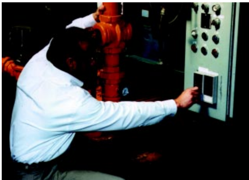
Keith Carter adjusts the setpoint of a Siemens Moore draft controller at Boiler No. 2 in the Wilson Sporting Goods plant in Humboldt, Tennessee.
