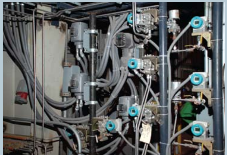
More than 30 SITRANS pressure and temperature transmitters are connected by PROFIBUS PA to the PCS 7 system.
