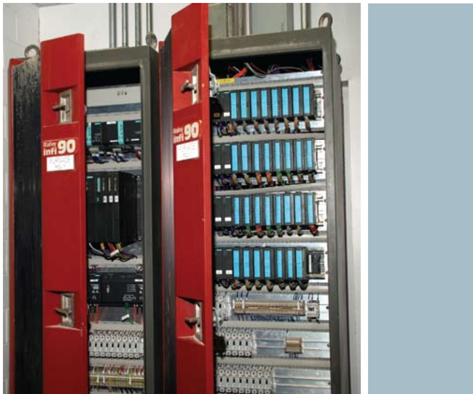
Cardinal Glass engineers say a big reason the Menomonie plant met its cold repair schedule was because they saved time by retrofitting the existing Bailey control cabinets with new PCS 7 hardware.
