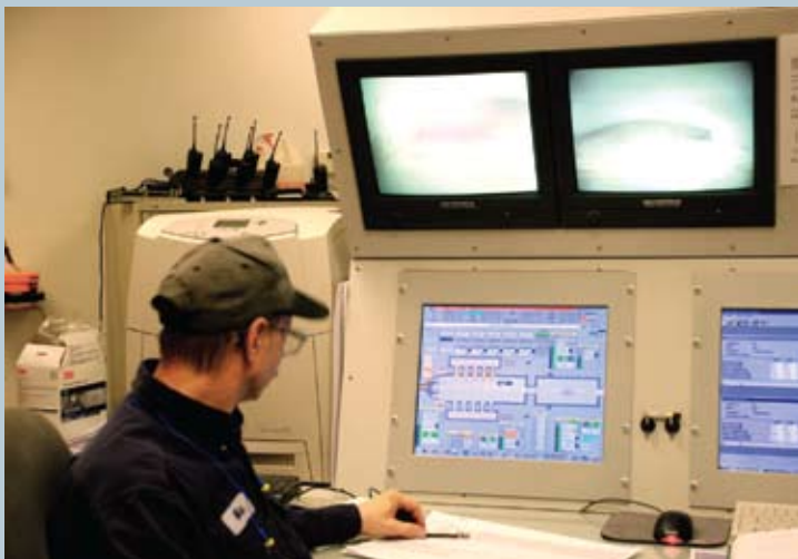
Operators in the central control room use video to monitor a furnace that is maintained at target temperature by the PCS 7 system.
