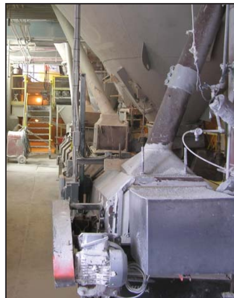
Figure 3. A 2-hp SE&A IEEE Plus belt conveyor motor (lower right of photo) that transports finely-ground product to the beneficiation department. It was one of the first copper-rotor motors installed during the current replacement program. The data plate lists the motor's NEMA nominal efficiency at 87.5%, one full percentage point higher than called for under NEMA Premium standards.
