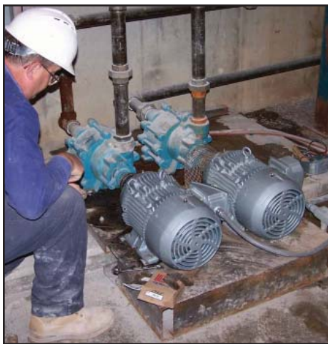
Figure 4. An electrician installs two new copper-rotor 10-hp SE&A IEEE Plus motors that will supply boiler feedwater for process steam. The SE&A motors are rated for a NEMA nominal efficiency of 92.4% at 100% load factor, which exceeds the NEMA Premium requirement by 0.7 percentage points. Tests conducted for CDA show that a copper-rotor SE&A motor of this size actually displays an efficiency of 92.72% at full load and greater than 93% at a 75% load factor.
