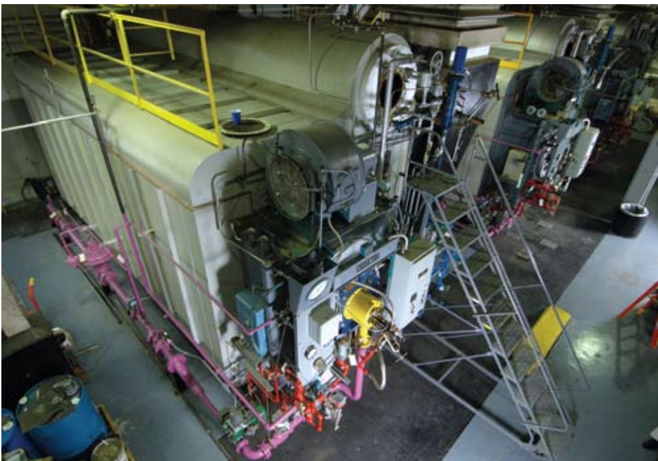
Overhead view of the three boilers at Ellis Hospital.
