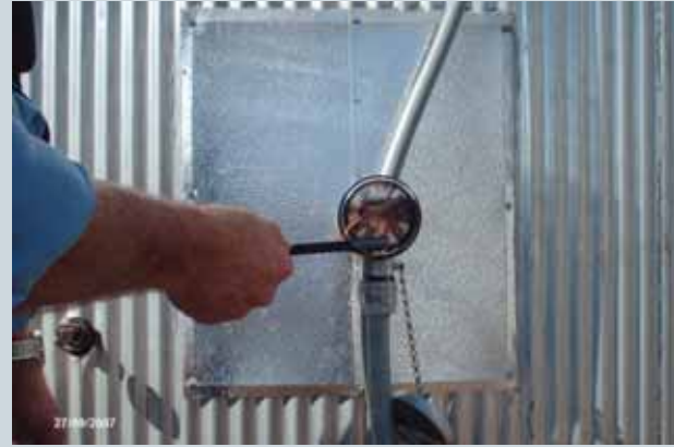
Fig. 10: Temperature transmitter incased in water
