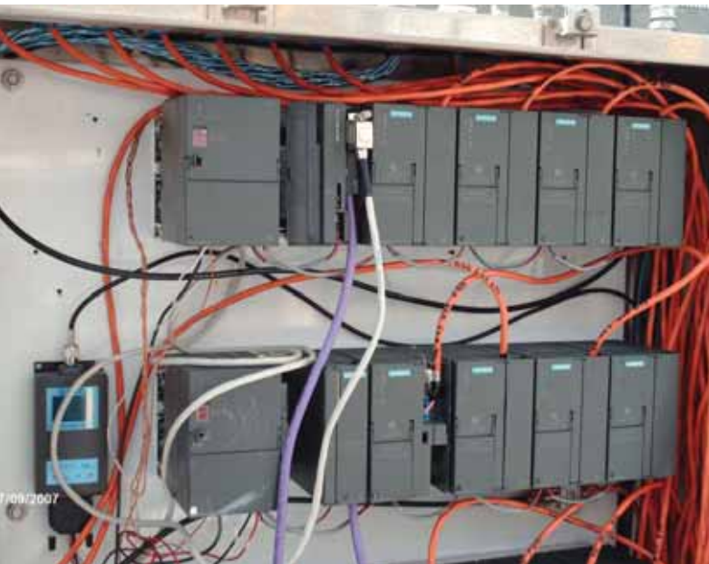
Figure 3: One of the panels shows violation of Profibus DP wiring guidelines
